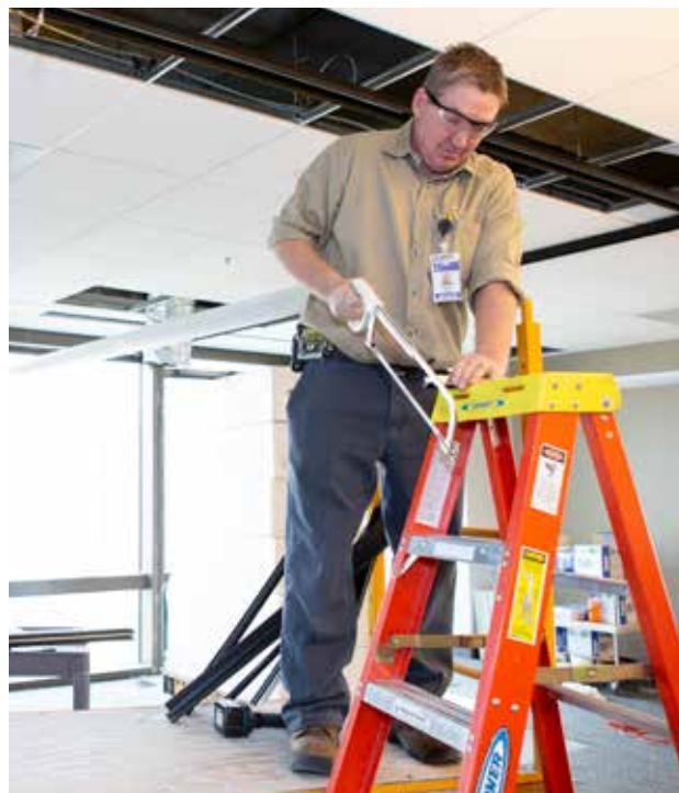
Senior Technician Steve VanDee of Facilities Management works on improvements at the Bank's headquarters.
